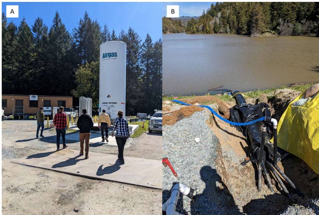
Figure 8.4.1.2. A) Onshore elements of a HOS installed in Loch Lomond, Santa Cruz, CA; B) Pipes connecting the onshore elements with the diffusers in the lake
